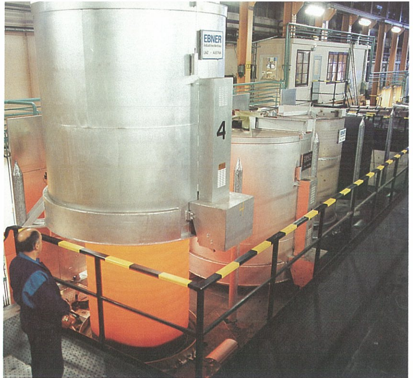
New bell furnaces double capacity for annealing of steel strip used in the manufacture of razorblades and knives, for example.
