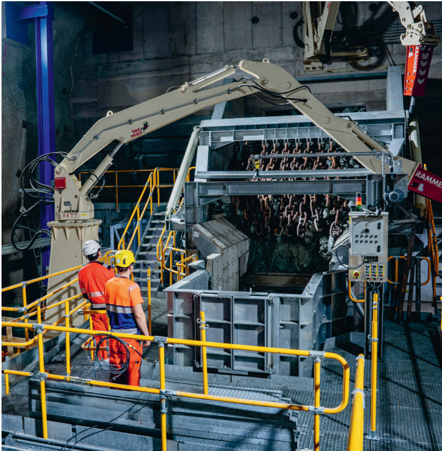
Crushing and screening are fully automated at the Wolfram mine.
