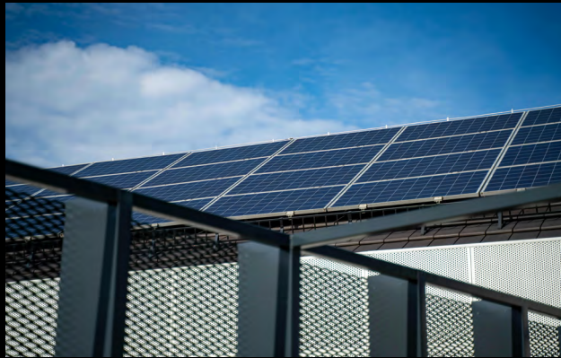
Expansion of rooftop solar installations
